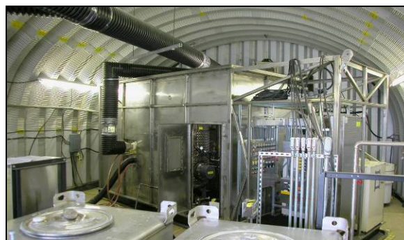
Exterior of LITANS Process Skid
